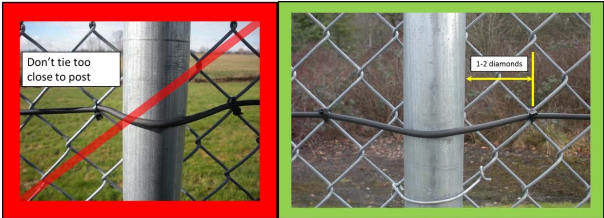
Figure 2-4. Do not tie the cable to the fence too closely to the fence posts.
